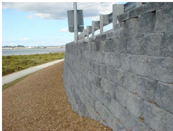
Firth retaining wall adjacent to MHX project using Diamond Pro bevelled retaining blocks in Rockface.
