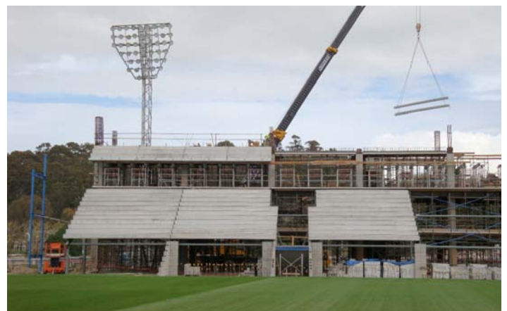
The South stand of the new Northland Events Centre , Whangarei, begins to take shape. Busck are supplying the entire Precast package including stairs, panels, bleachers, flooring, beams and balconies.
