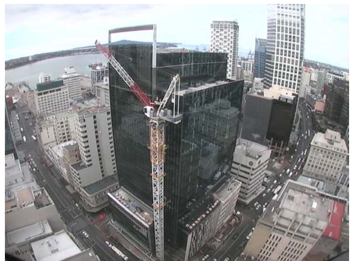
Deloitte Centre, Queen St. Currently nearing completion by Brookfield Multiplex. Precast Stairs by Busck.
